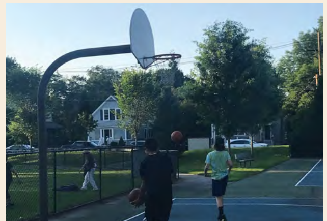
Basketball courts at Rideout and Emerson Parks are popular but contain cracks in the field of play, which should be repaired.
